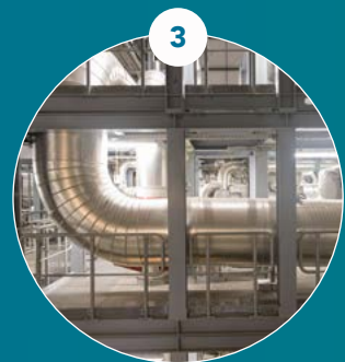
3 Flue gas treatment
